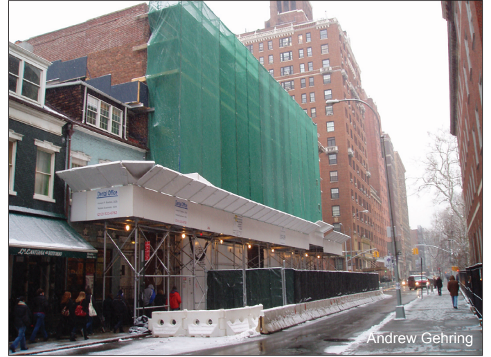
Construction has begun in earnest on the building at 135 Macdougall Street, formerly low-rise housing for students at the law school. The unit was closed down last spring so that renovations could take place. The overhaul coincides with other University-construction for the implementation of a cogeneration power system.
